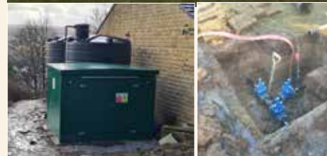
Improvements being made to Branshaw golf course to mitigate climate change and safeguard the facilities for the future.
